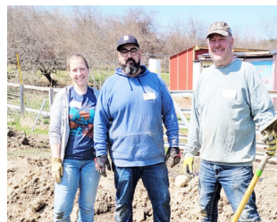
The Romeo Lions Club spent the day on April 22 at the Skyline Camp and Retreat Center in Almont assisting with readying the cabins for the season and with installing a French drainage system. Pictured here are Lion Richelle Lucero, Romeo Lions Club President Jamie Lucero, and Lion Larry Rekar
