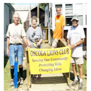
Lion ramp builders, Tony Priebe, Gov. Bill Gaines, John Novak, Ann Bovan and Chuck Andrina built a ramp for a home owner on Indian Trail. The ramp consisted of a 4x4 platform , 12' of ramp, a 4x8 platform and then another 28' ramp. Materials were paid for by the Homeowners family. The lady is currently using a walker but anticipates needing a wheelchair in near future.
